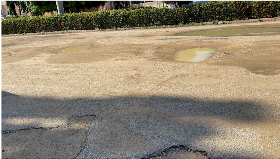
Image 2: A commercial area road with several potholes and stagnant water
