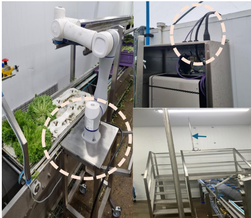
Figure 29 Harvesting room electrical and mechanical adaptation
