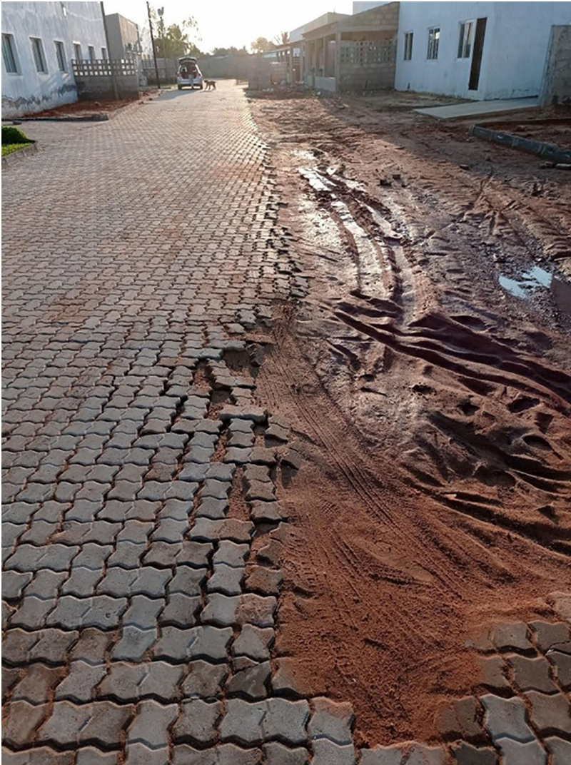
Figure 2. Paved road left unfinished due to the lack of contributions from some of the home owners. Photograph by Jason Sumich, July 2022.
